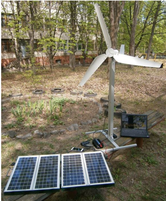
Fig. 1. Mobile combined photovoltaic / wind power station
